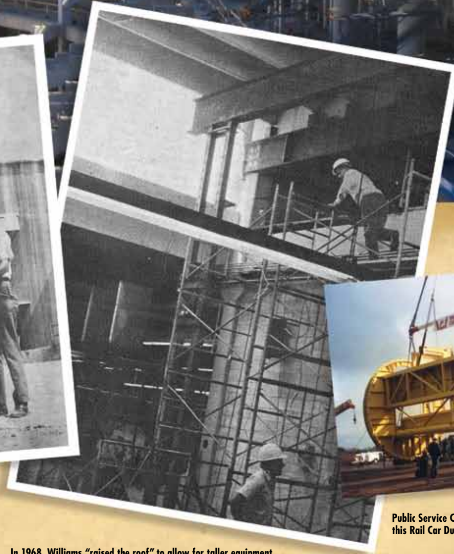
In 1968, Williams "raised the roof" to allow for taller equipment to be installed for the Mid-America Yarn Mill.
